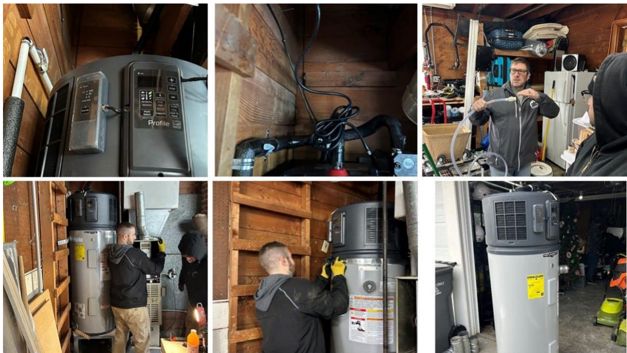
Images from AWHI's first installation of a flexible voltage HPWH in February 2026.
